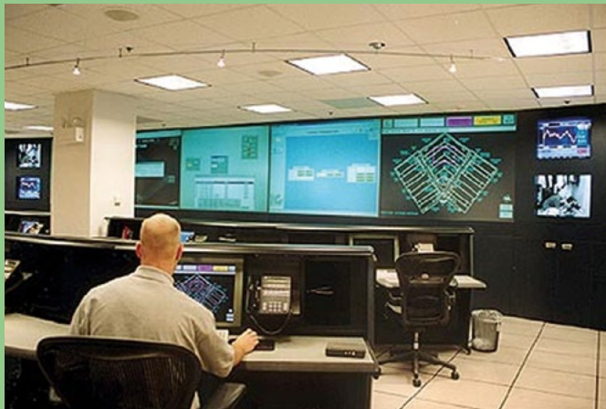
The Pentagon Building Operations Command Center
