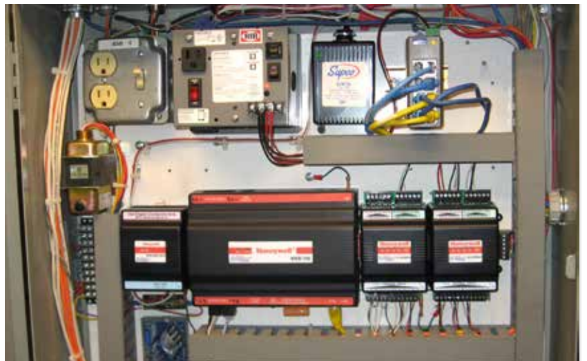
WAC's old analogue energy control system (top) was replaced by modern network-based digital controls (bottom)
